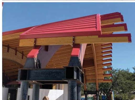
Top and right: Reusing the truss design, in a radial fan on two arches, similar to the roof design observed at the Main Stage (below).
